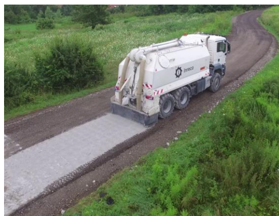
Figure 2 The process of stabilizing the base soil with cement in the field [2]
