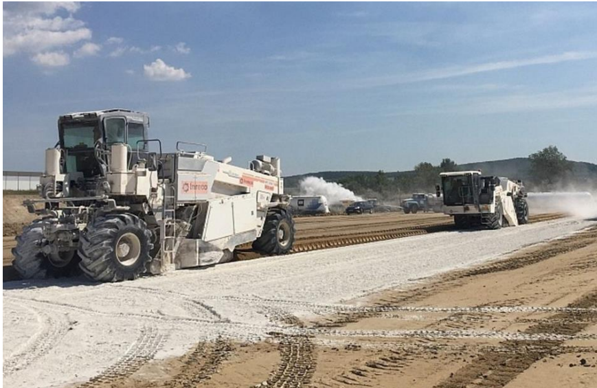
Figure 3 The process of stabilizing the base soil with lime in the field [2]
